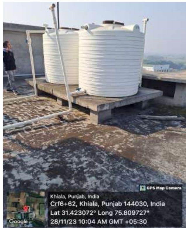
Rooftop plastic Water Tanks
