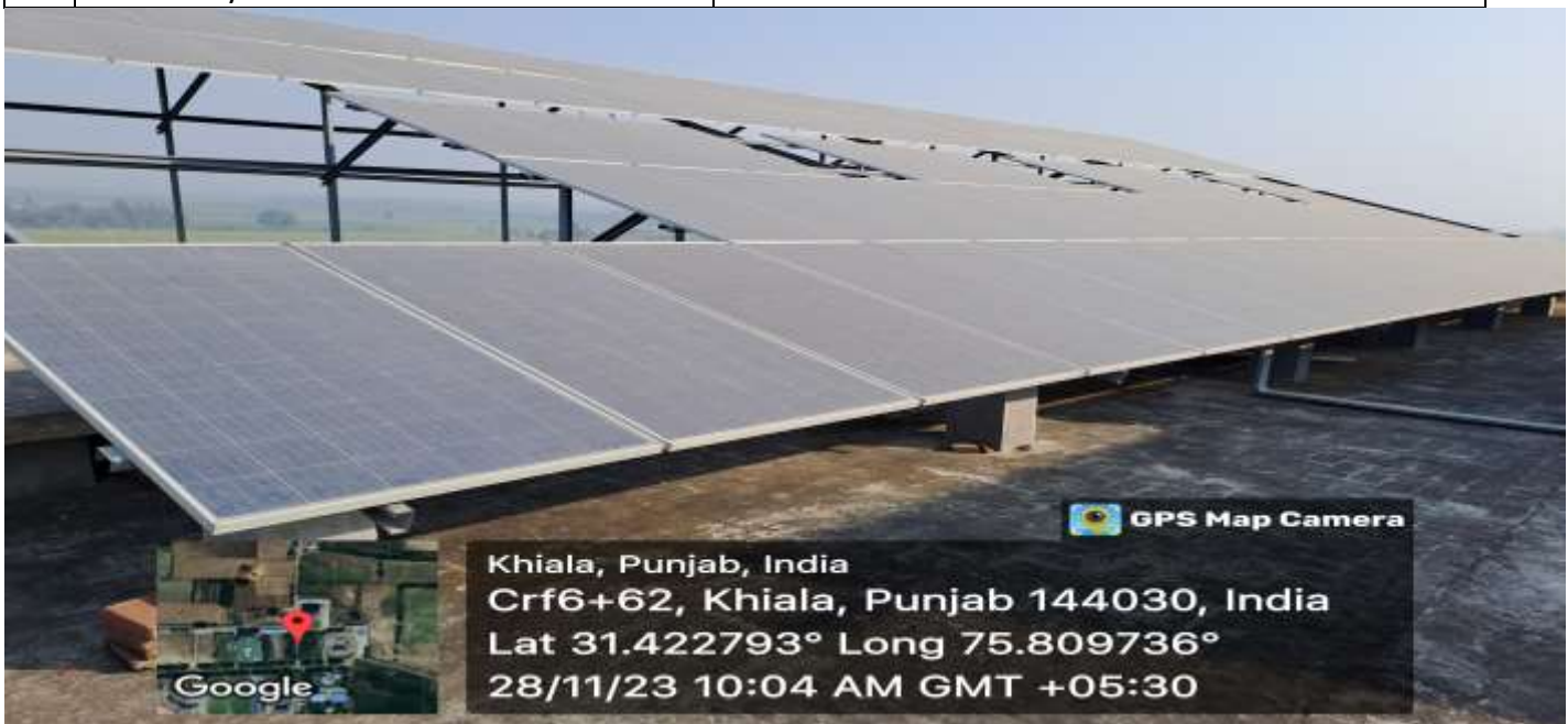
Rooftop Solar Power Plant At SBBS University, Jalandhar
