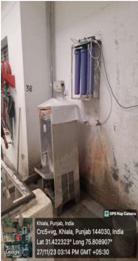
Existing RO FILTERS in the campus
