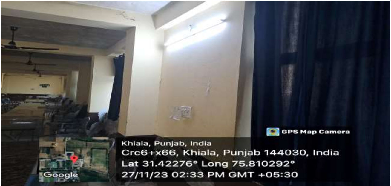
Conventional FTL Are Being Replaced with Energy Efficient LED Lights In Campus
