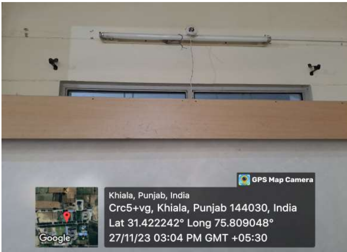
Existing FTL 40 watts installed in the campus ←
