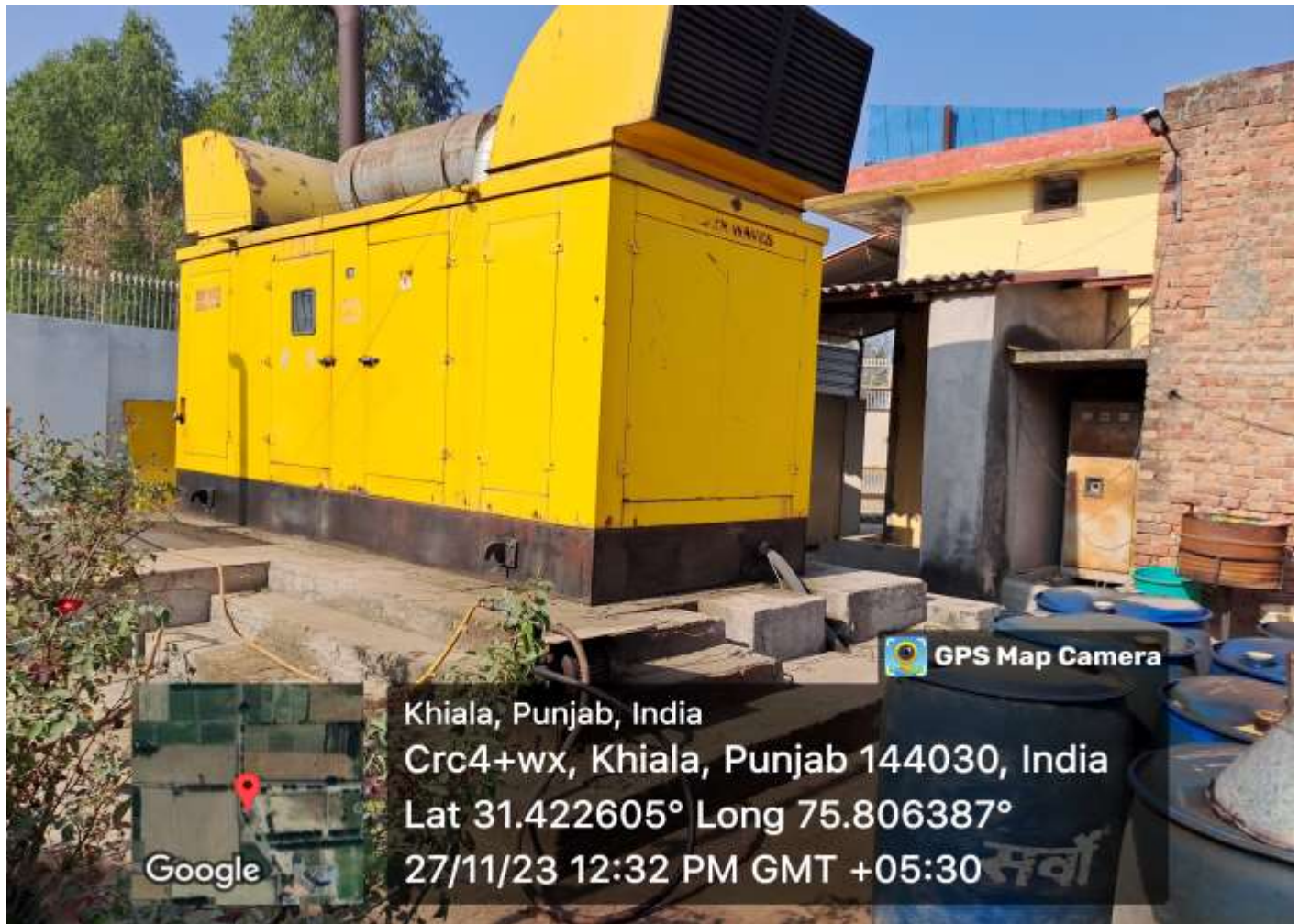
Existing DG Set 500 KVA installed in the university
