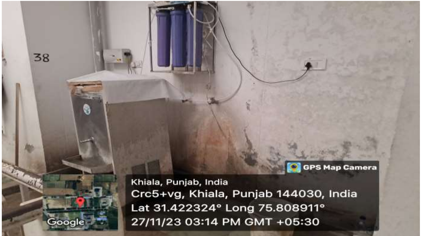
Existing water cooler in the campus
