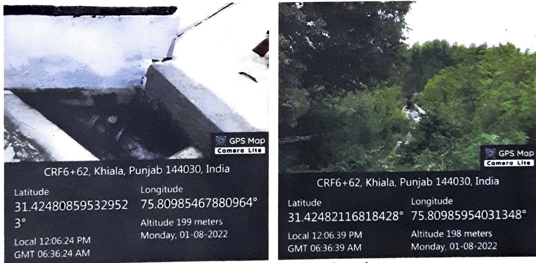
Figure 5: Clean water coming out of STP and supplied to plantation purpose
